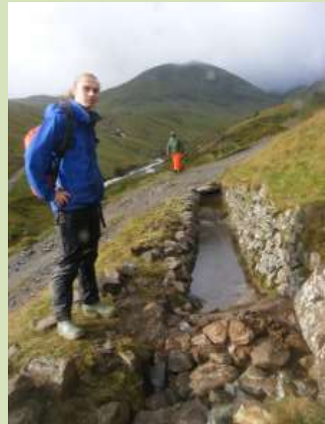
Old leet at Greenside mine near Glenridding Common cleared and wall was later repaired
