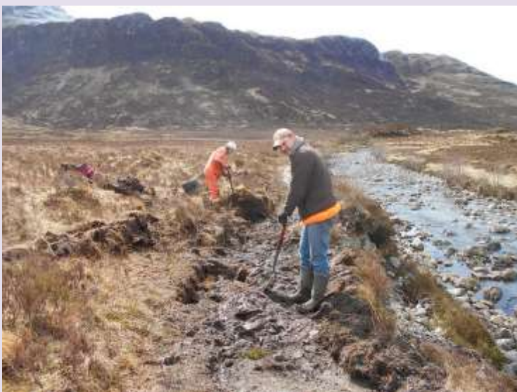
Building a new section of path to Mam Li away from river (on Knoydart)
